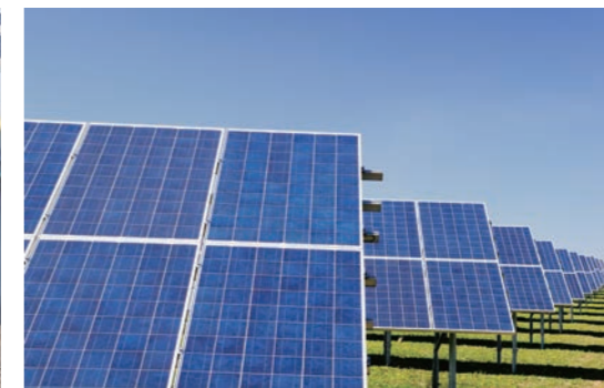
Ground Power Station Scene
